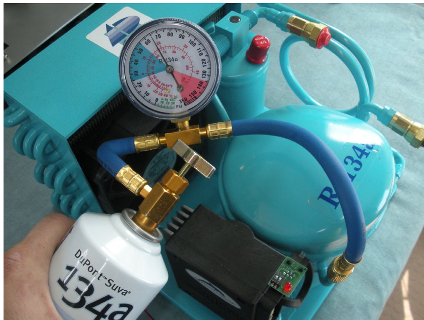
Figure 33: Compressor Recharge Port for Adding Freon
